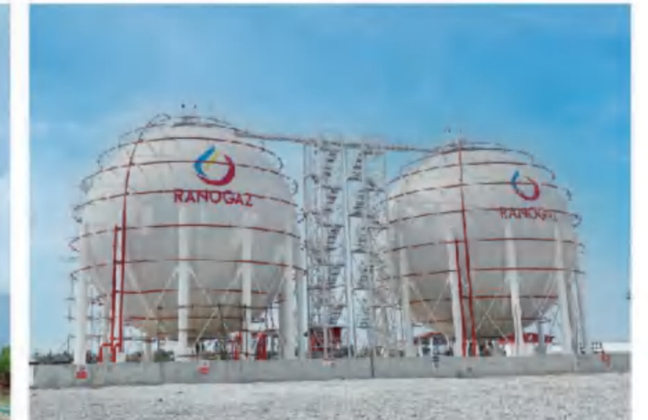
Nigeria 2x5000m 3 Spherical Tanks
