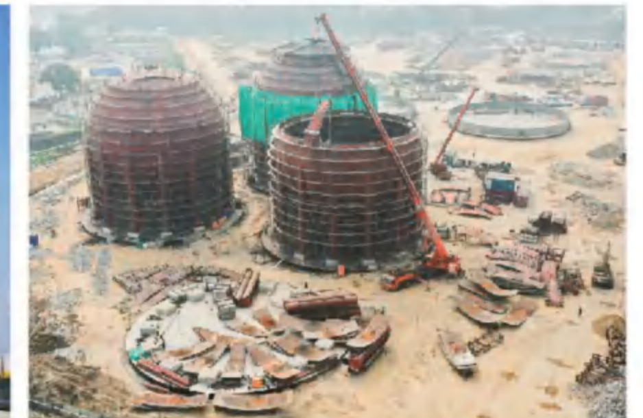
Nigeria 4x10000m 3 Spherical Tanks
