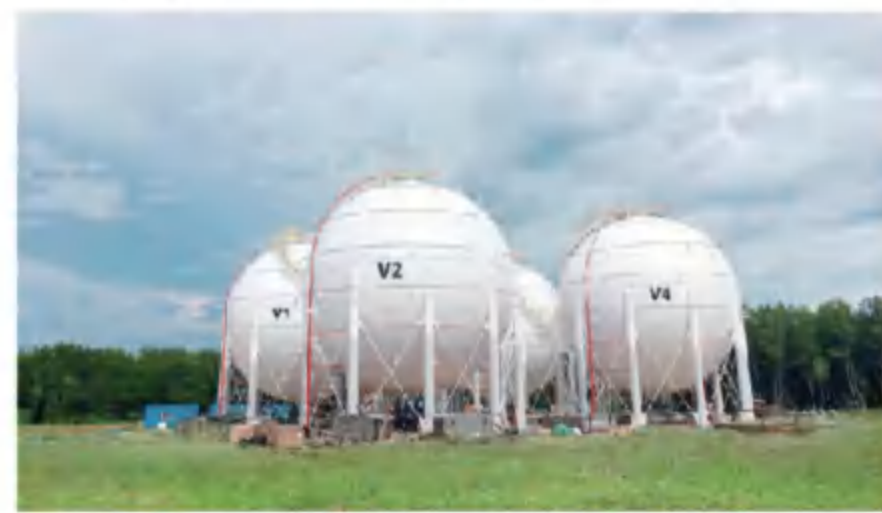
Thailand 4x2000m 3 Spherical Tanks
