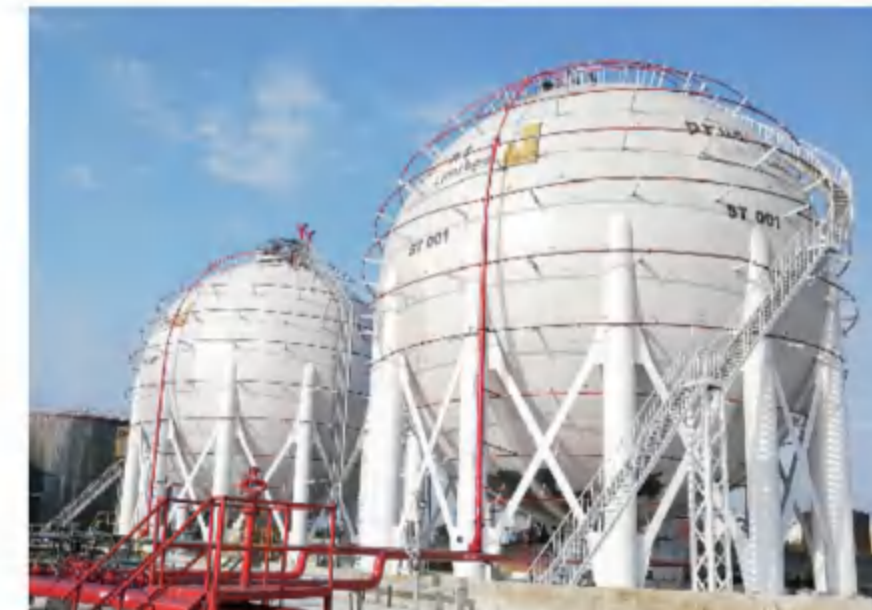
Nigeria 2x6000m 3 Spherical Tank
