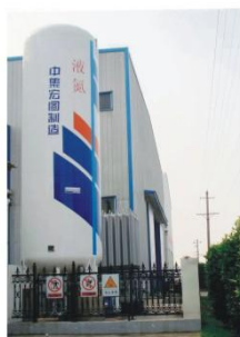
液氮储罐 Liquefied nitrogen storage tank
